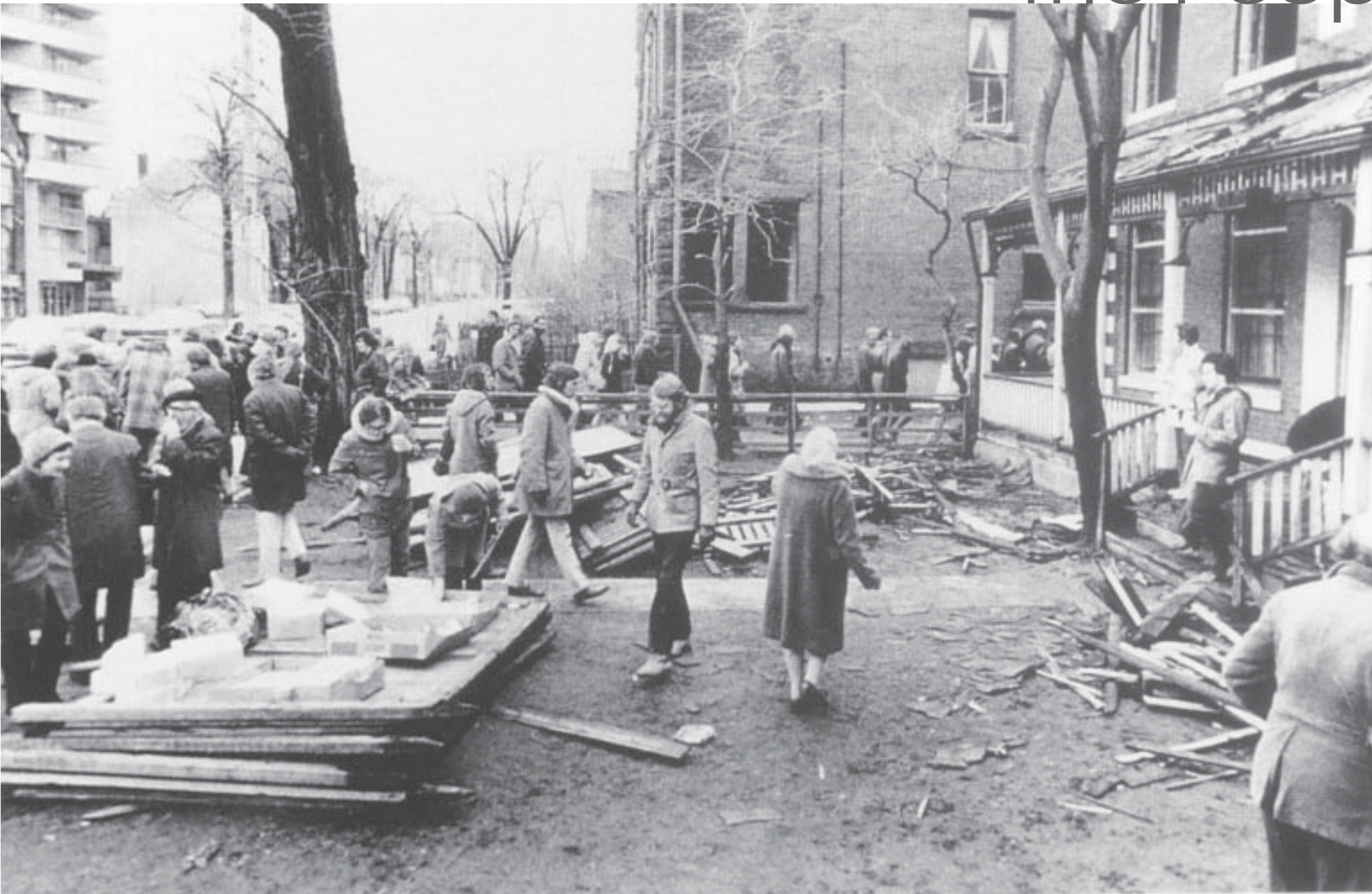
April 5, 1973 Protesters halted demolition of the old houses and forced the City to offer alternatives to eviction for construction of high-rise housing.
